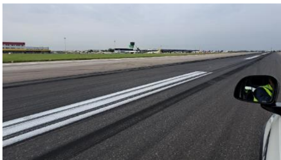
Photo 4 - skid marks on the runway
