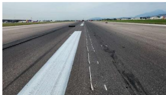
Photo 5: runway damage and debris on the runway
